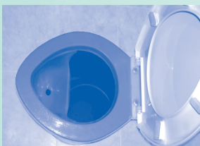
Photo: Self-made cement urine diverting toilet used in rural areas of Eastern Europe is hygienic and prevents groundwater pollution
