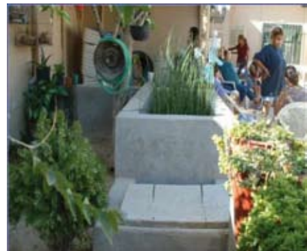
A wetland filter cleans household wastewater
