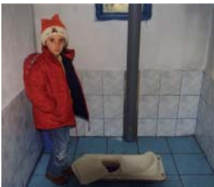
EcoSan toilets in Garla Mare, Romania
