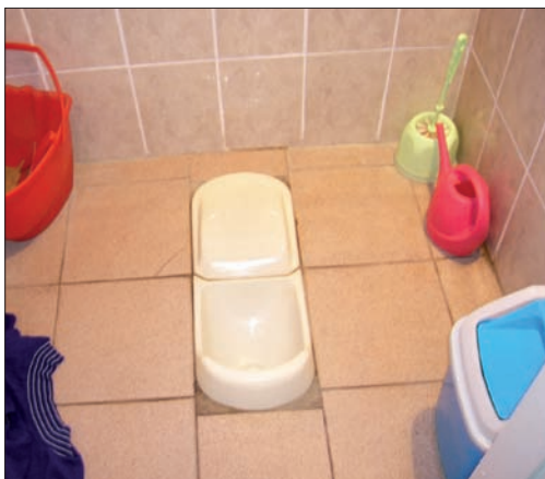
Vas WC in interiorul camerelor toaletei (tip turcesc)
