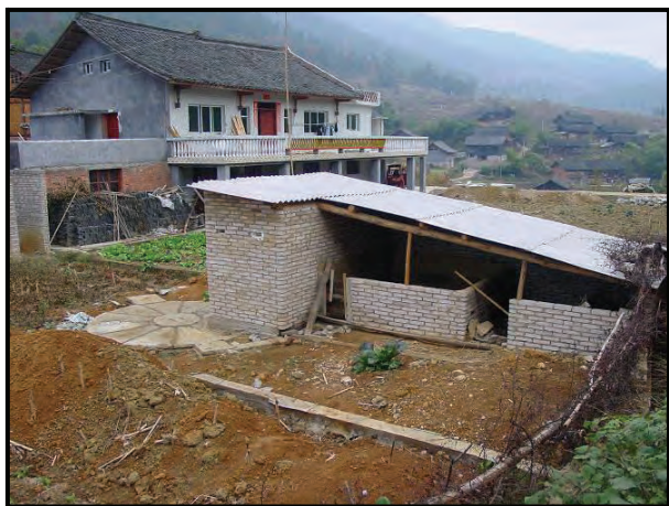
A biogas tank and pigsty once finished
