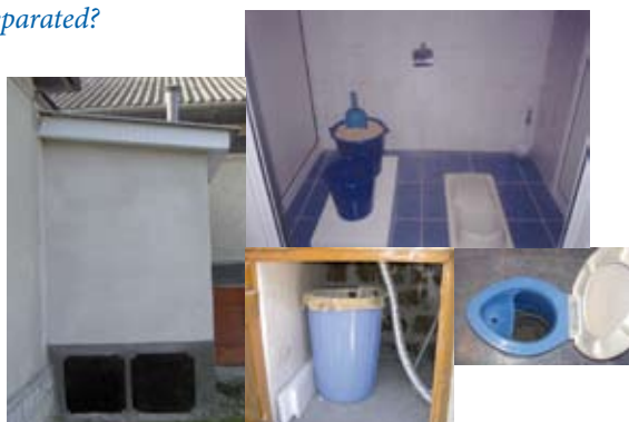
Separation and storage of faecal matter of ecosan toilet
