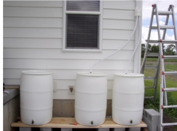
Rain water barrels
