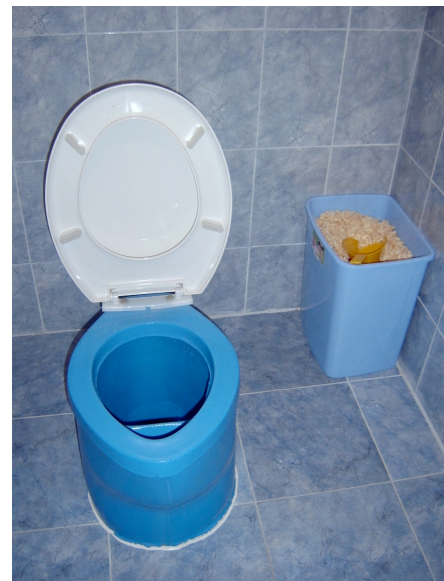
Interior of an Ecosan toilet, toilet (UDDT), constructed inside of a house in Bulgaria. Photo Earth Forever
