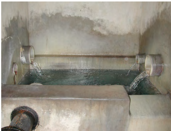
Water collection of a spring in Bavaria. Tapping of the spring can be carried out with several drainage pipes. The basin should be covered and ferment proof.
