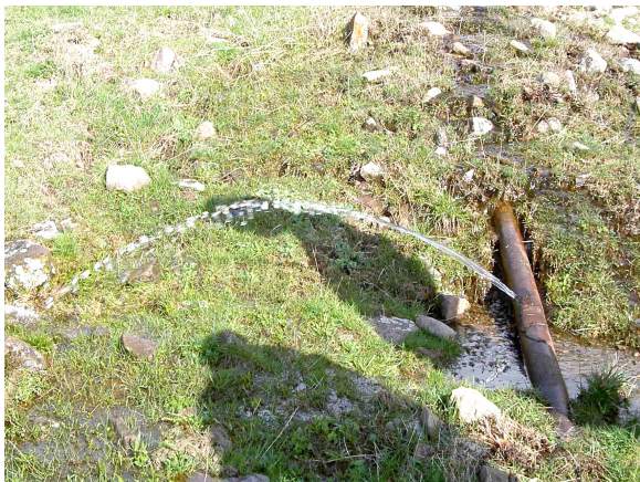
Corrosion can cause severe leakages in the distribution system
