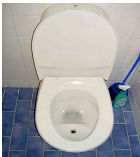
Urine diverting toilet with water flush
