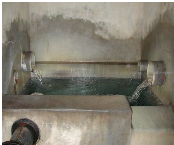
Water collection of a spring in Bavaria. Tapping of the spring can be carried out with several drainage pipes. The basin should be covered and ferment proof.
