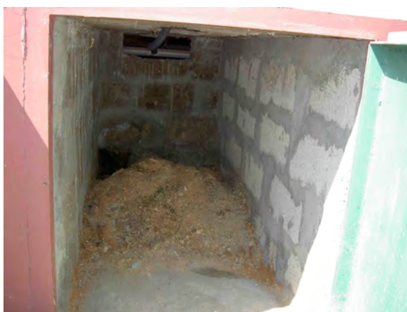
School UDDT: chamber for the collection, storage and treatment of faecal matter
