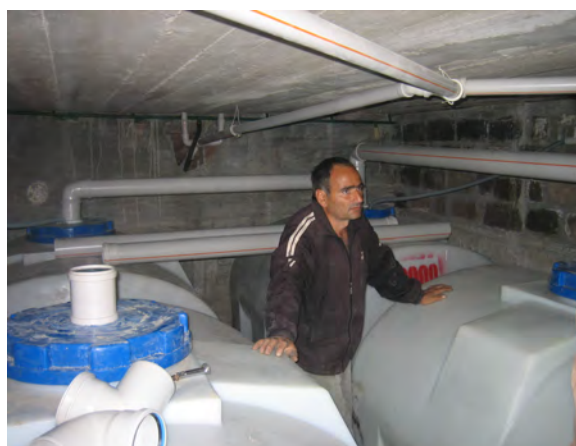
School UDDT: basement with reservoirs for the collection, storage and treatment of the urine of 350 users
