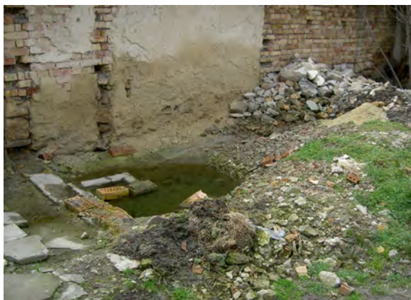
A soak away pit filled with wastewater
