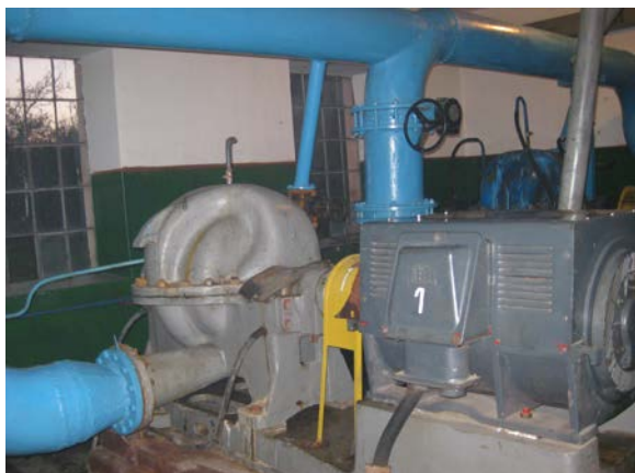
Engine room at the water supplier
