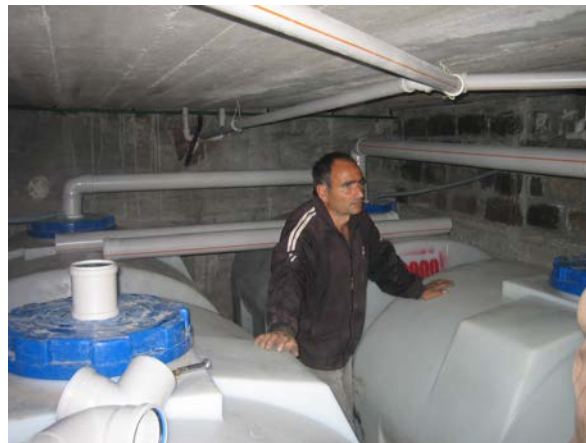
School UDDT: basement with reservoirs for the collection, storage and treatment of the urine of 350 users
