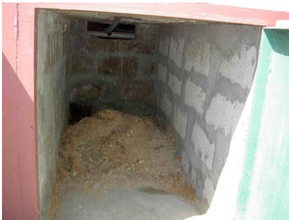
School UDDT: chamber for the collection, storage and treatment of faecal matter
