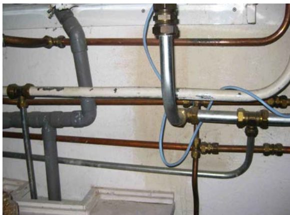
The purpose of the distribution within the house will influence the selection of the materials
