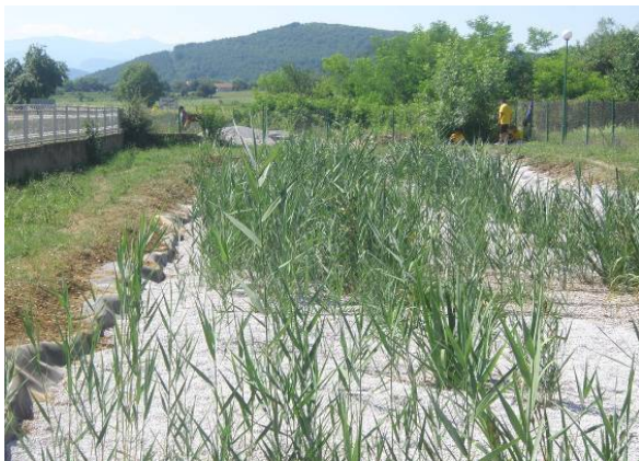
Soil filter with planted reed in Vidrare
