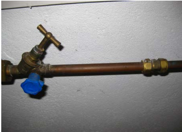
Copper pipes are characterised by durability and reliability, but are relatively expensive.
