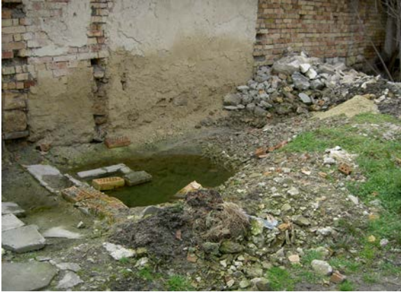
A soak away pit filled with wastewater
