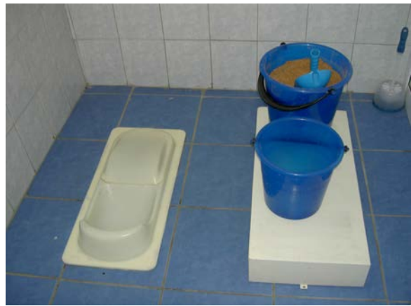
Interior of a UDDT for a school
