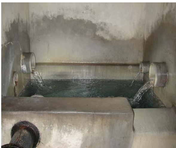
Water collection of a spring in Bavaria. Tapping of the spring can be carried out with several drainage pipes. The basin should be covered and ferment proof. Photo source: Bayerisches Landesamt für Umwelt (Bavarian State office for Environment); http://www.lfu.bayern.de/wasser/merkblattsammlung/teil2_gewaesserkundlicher_dienst/doc/nr_219_anlage6.pdf
