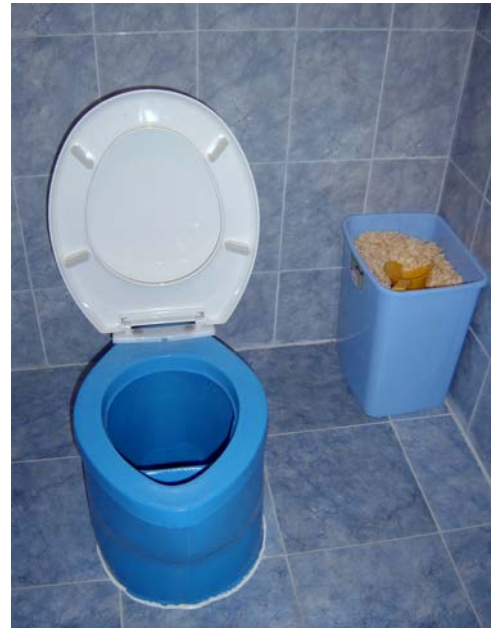
Interior of an Ecosan toilet (UDDT) cabin, constructed inside of a house in Bulgaria. Photo: Earth Forever
