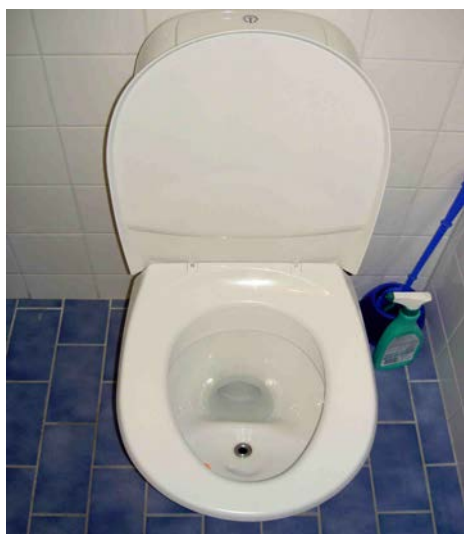
Urine diverting toilet with water flush
