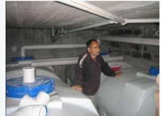
Urine storage tanks in the basement
